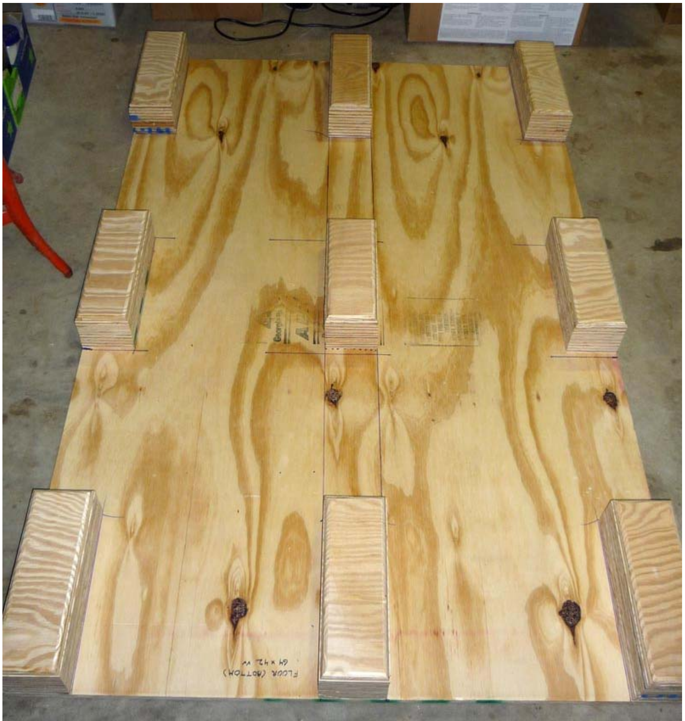
Caption: An additional 1/2" layer of plywood was laminated to the floor. A second set of (27) 3" screws was installed from the top.
